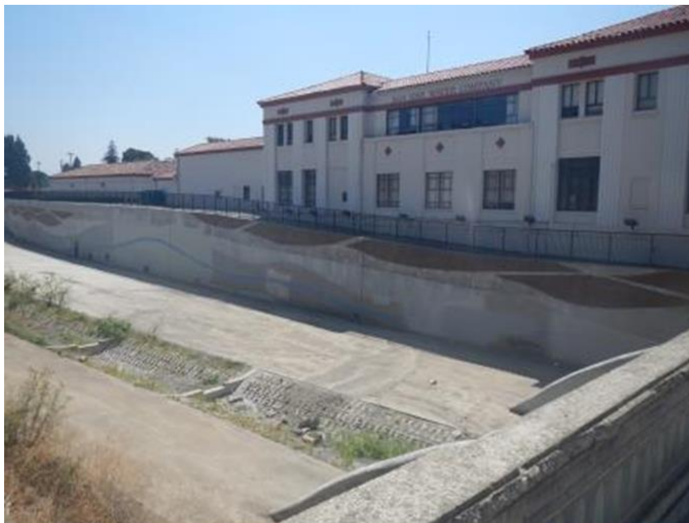
2. Concrete floodwall on west side of Guadalupe River abuts existing buildings at Project site.
